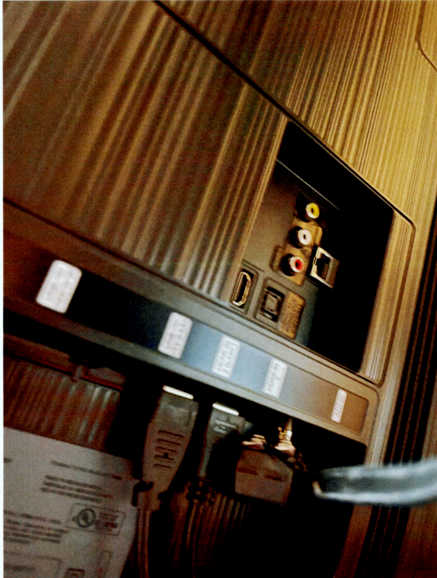
Figure 6: Cables Connected to TV with Ethernet port visible
